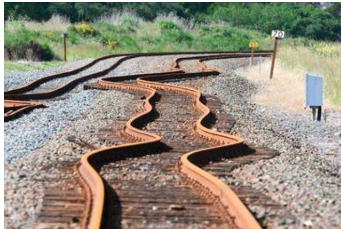
Figure 7.6 Twisted railway lines in the aftermath of an earthquake (Figure 5 in https://www.intechopen.com/chapters/60627 )
