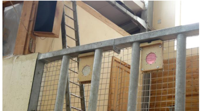
Figure 2: Shower buttons mounted on balcony
