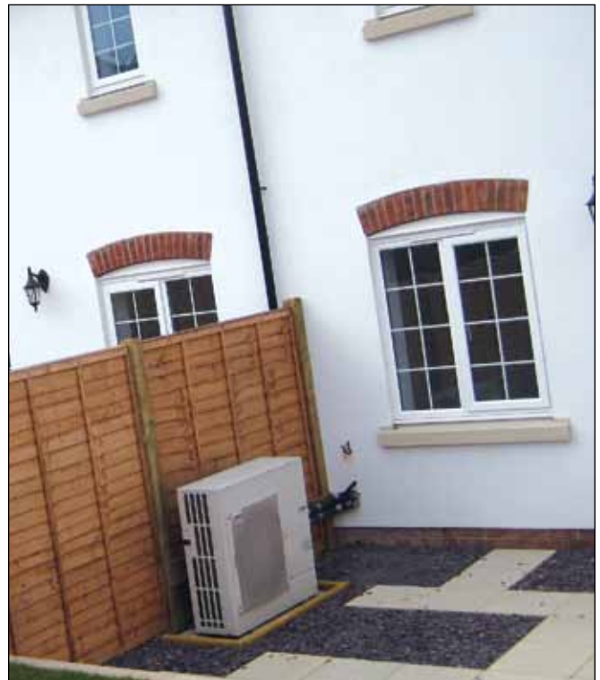
Air source heat pump
